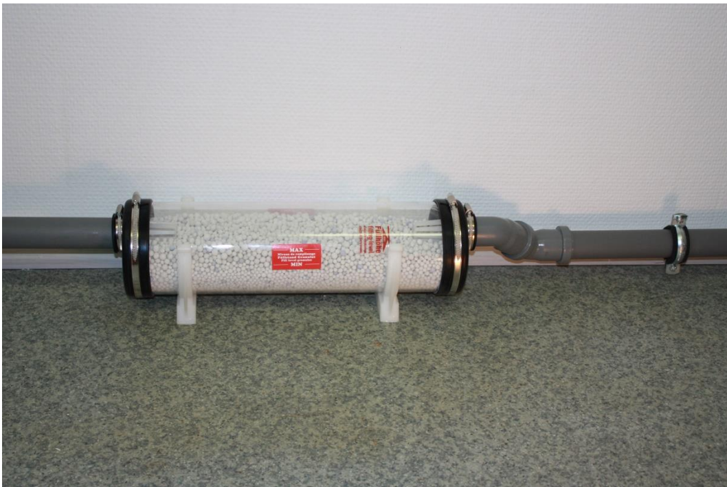
Abb. 6 / Neutralization mounted on the floor with inlet and outlet DN 40.
